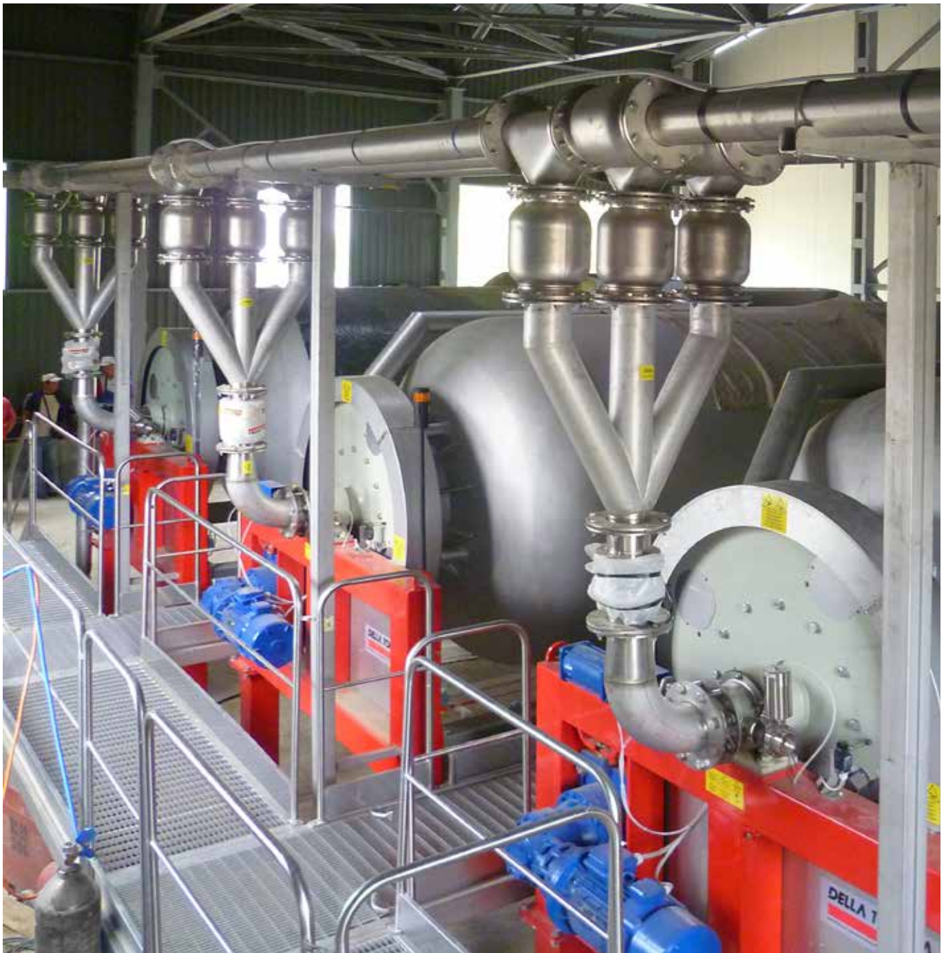
Closed-tank pneumatic press system, Moldova
